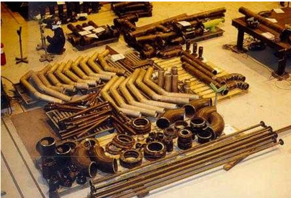
Example of stocking pipes and fittings, separating steel and stainless steel .
